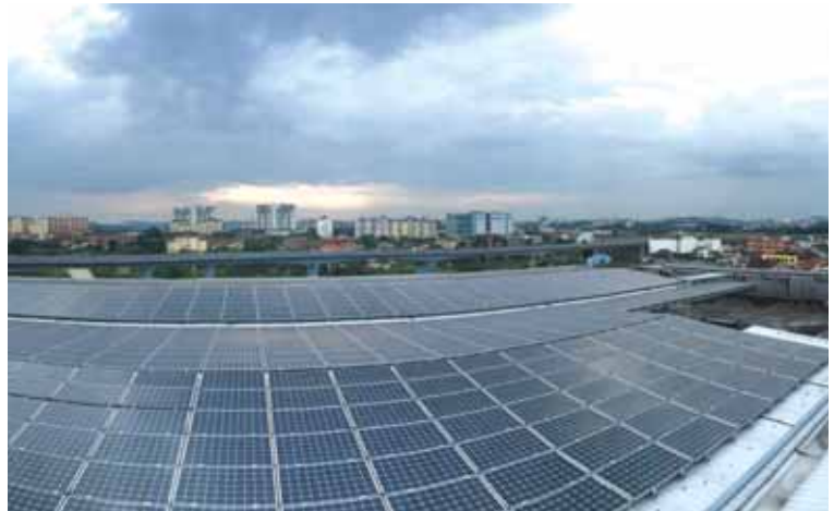
The solar photovoltaic panels installed on the rooftop of Plaza Metro Kajang is estimated to reduce electricity consumption by about 10% annually
